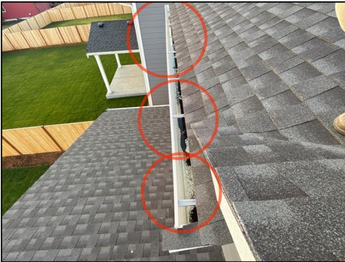
1. Improper slope, ponding
