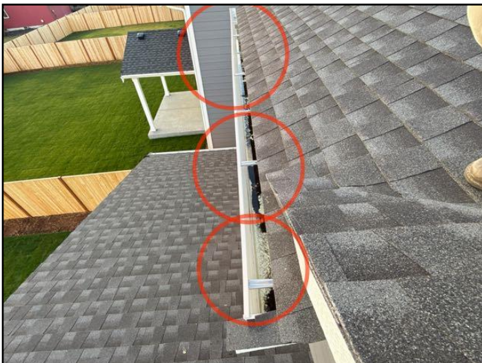
12. Improper slope, ponding
