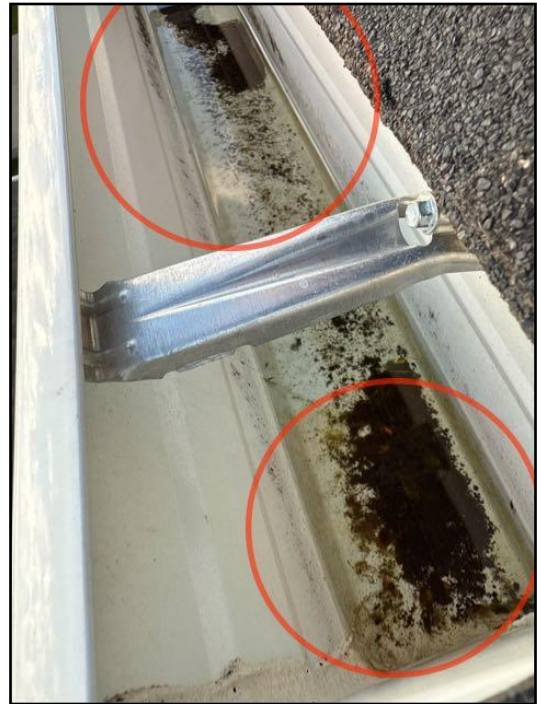
2. Improper slope, ponding
