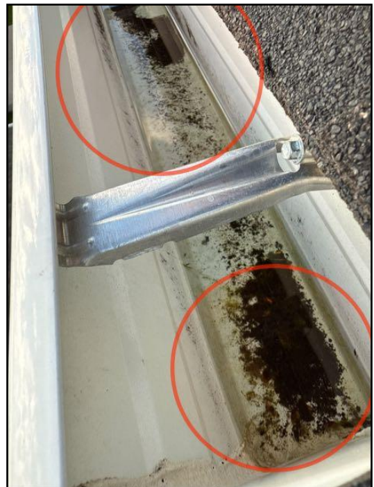
13. Improper slope, ponding
