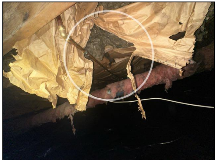
132. Loose, sagging or voids
