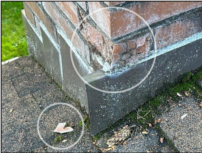
121. Loose, missing or deteriorated masonry
