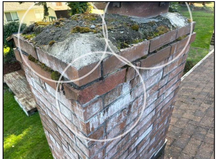
16. Loose, missing or deteriorated masonry
