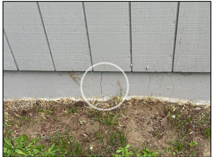
84. Typical minor cracks
