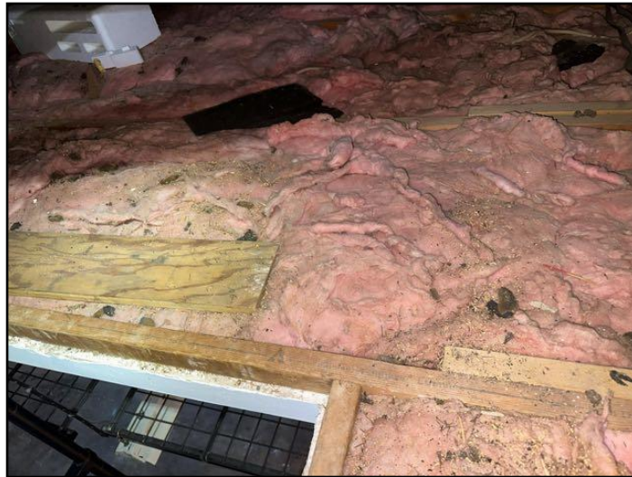
130. Animal/pest droppings in attic
