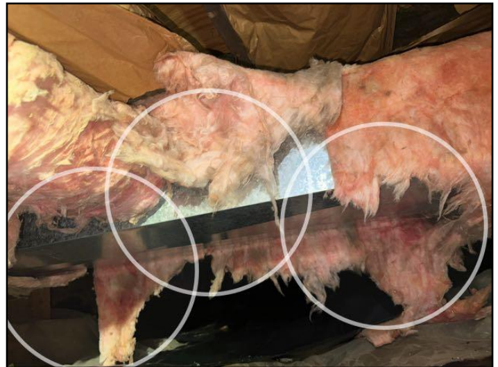
116. Insulation missing, damaged
