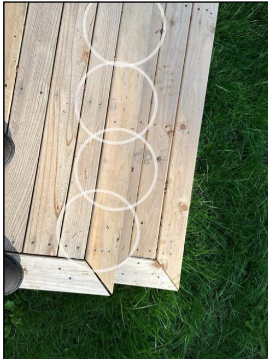
62. Loose deck board
