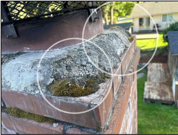
17. Loose, missing or deteriorated masonry
