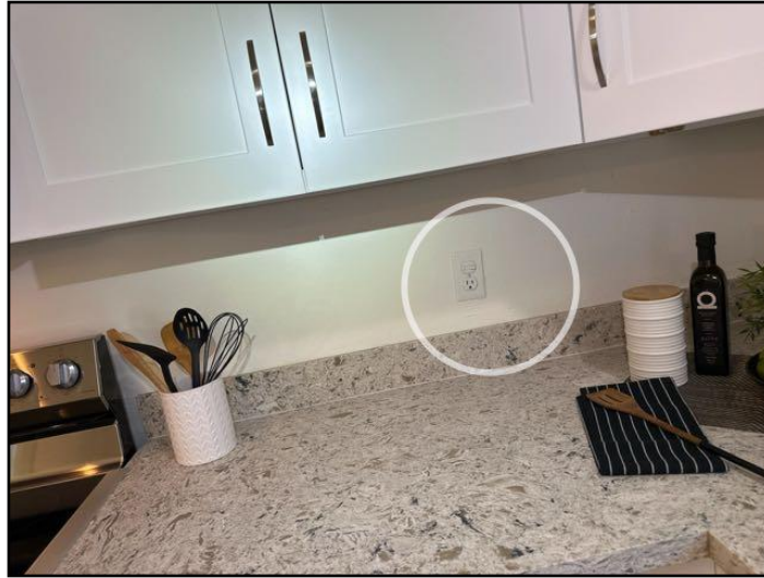
105. No GFCI/GFI (Ground Fault Circuit...
