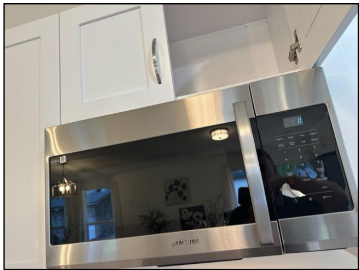
168. Not vented to exterior
