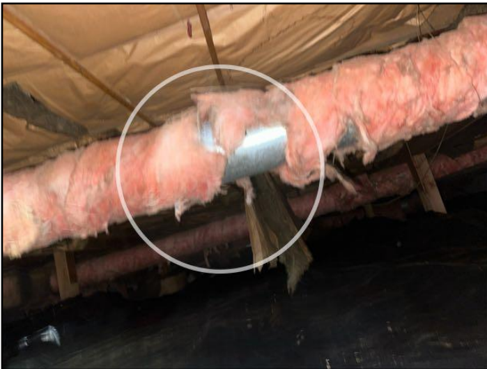
115. Insulation missing, damaged
