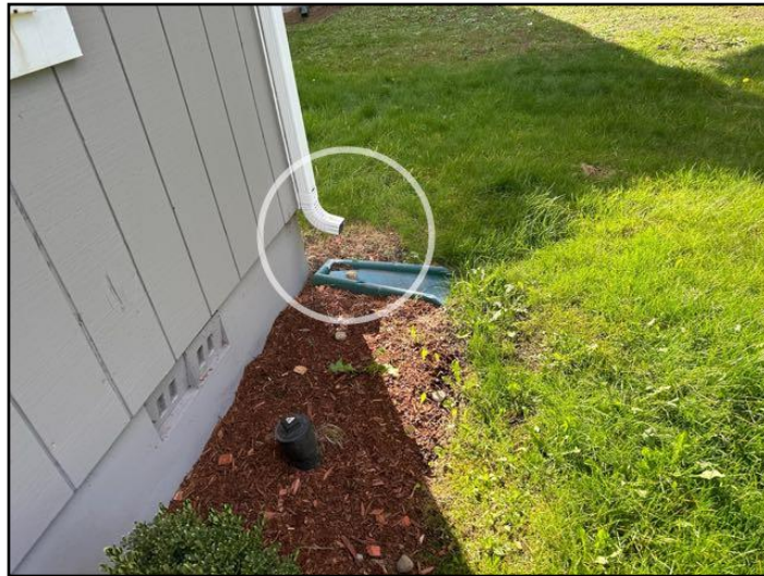
55. Discharge too close to building
