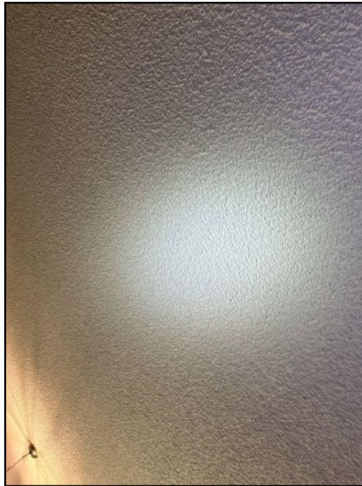
174. Possible asbestos containing materials
