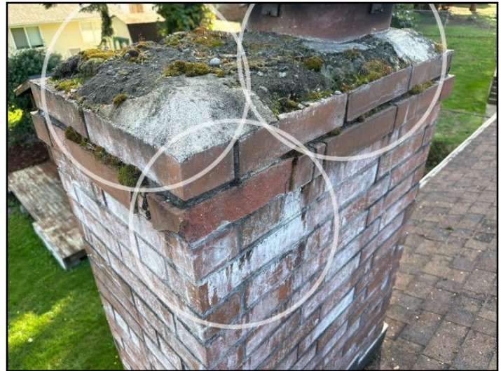
122. Loose, missing or deteriorated masonry
