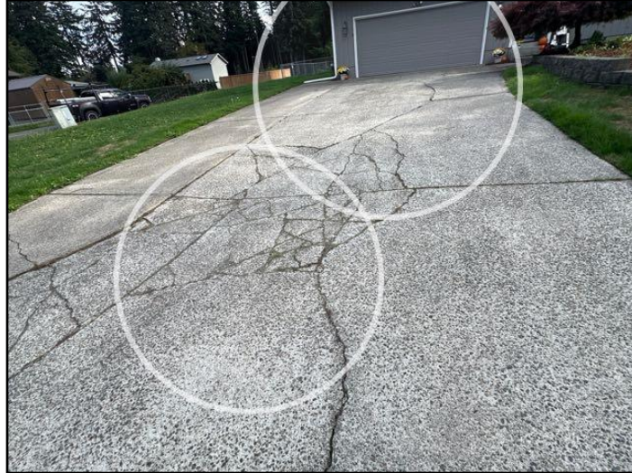
67. Cracked or damaged surfaces
