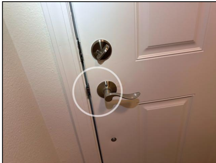
167. Latch not effective on exterior door
