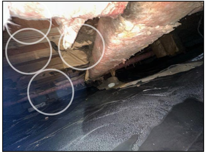
134. Loose, sagging or voids
