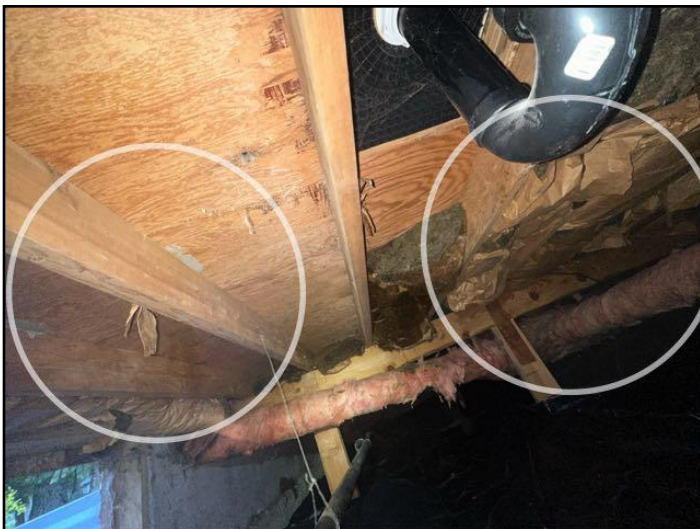
131. Loose, sagging or voids
