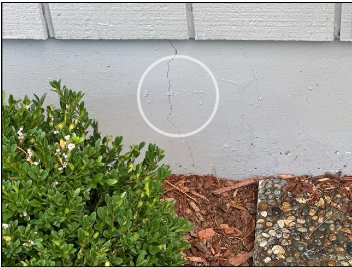
83. Typical minor cracks
