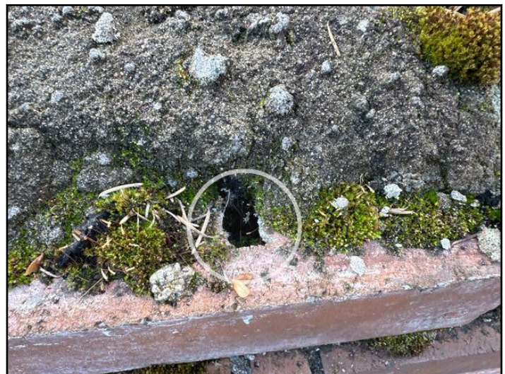
124. Loose, missing or deteriorated masonry
