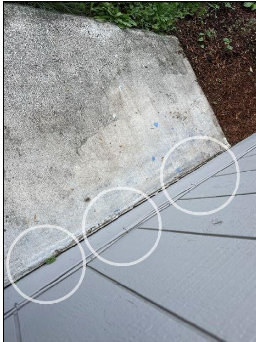
66. Unsealed gap at building
