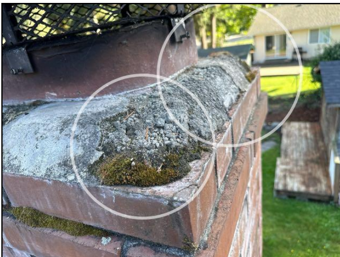
123. Loose, missing or deteriorated masonry
