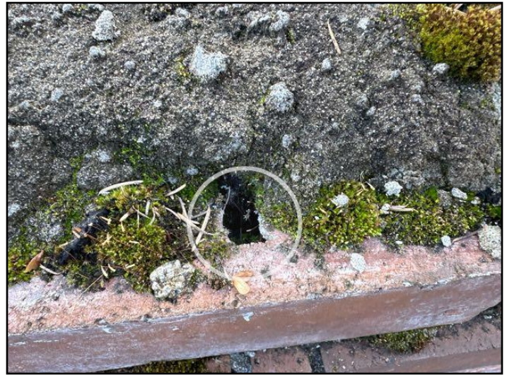
18. Loose, missing or deteriorated masonry
