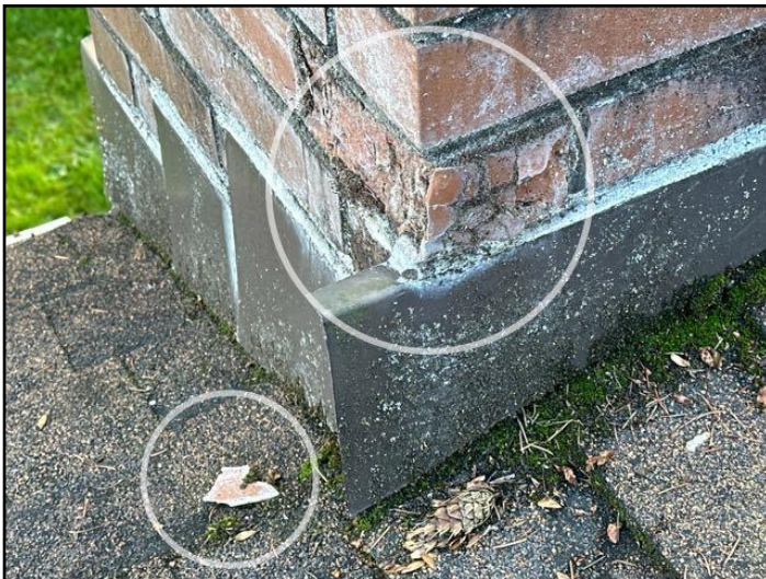
15. Loose, missing or deteriorated masonry
