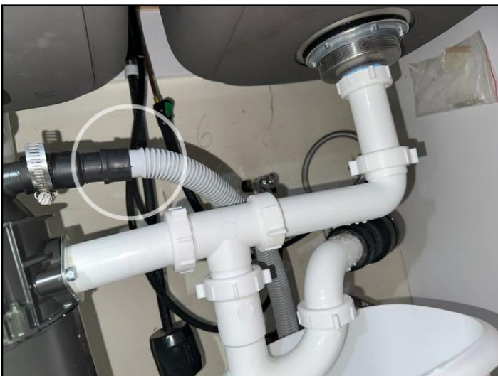
171. Backflow prevention high loop missing
