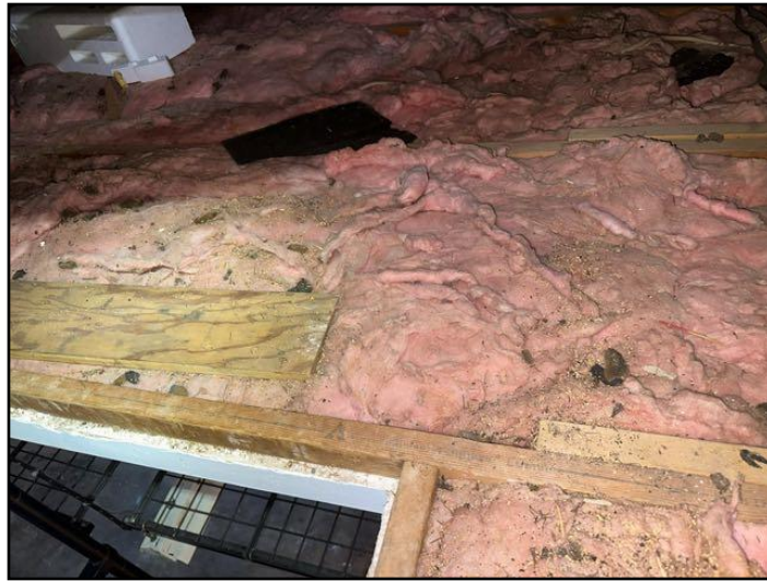
21. Animal/pest droppings in attic
