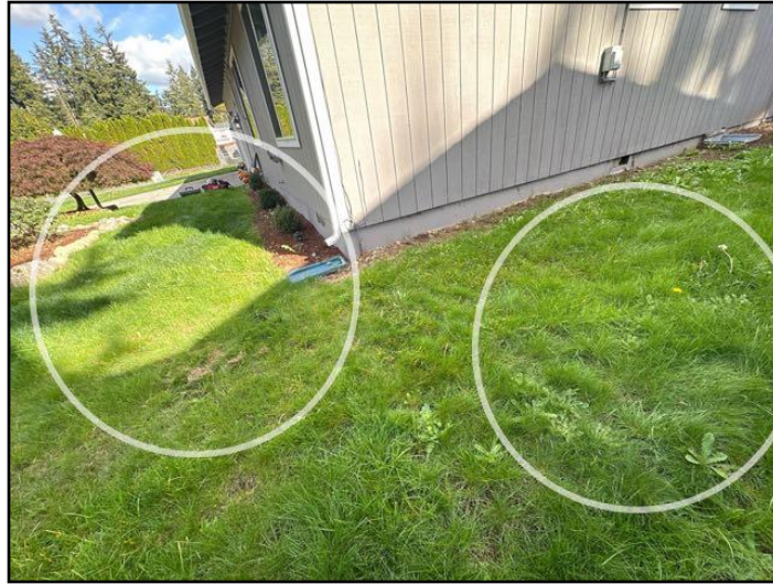
65. Improper slope or drainage
